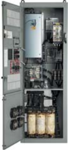
Enclosed 18-Pulse Drive
